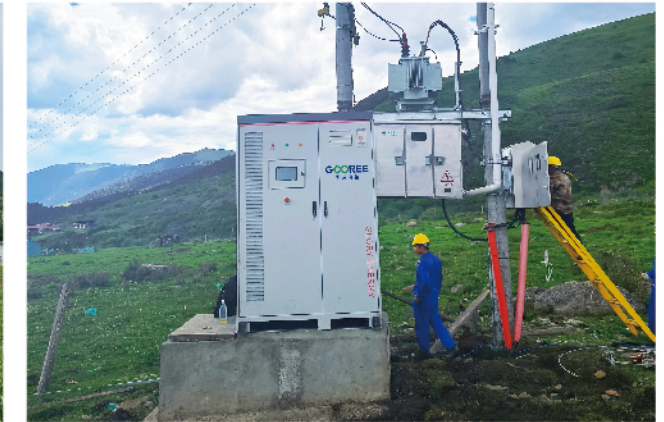
Distribution Energy Storage
