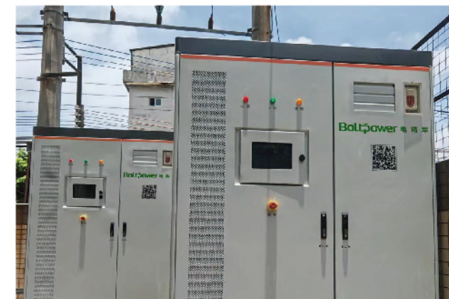
Transformer Capacity Expansion
